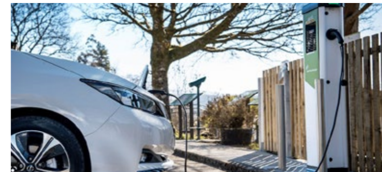
5. EV charging points
