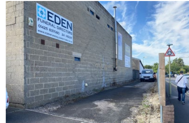
2. Poorly finished buildings and space in need of upgrade
